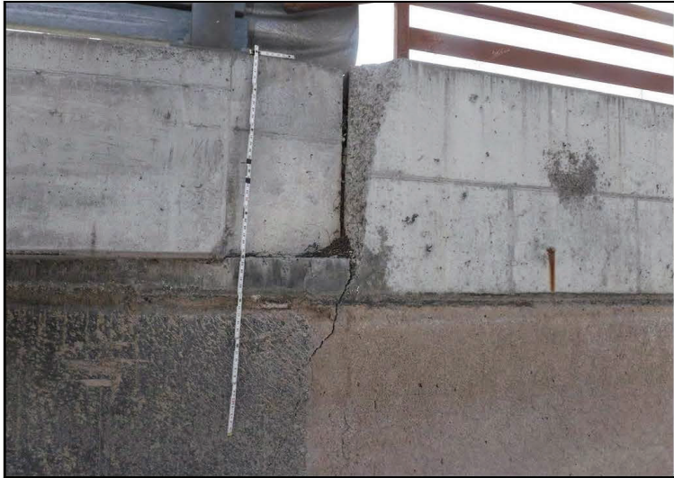
Spall and vertical crack in northwest wingwall
