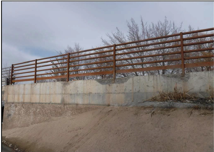
Spalls in southeast wingwall at rail posts
