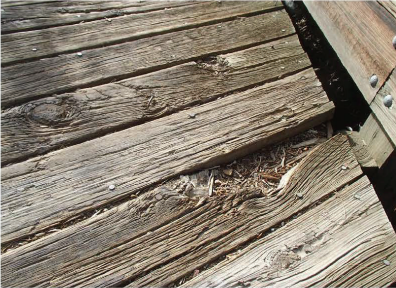
Rotted deck plank
