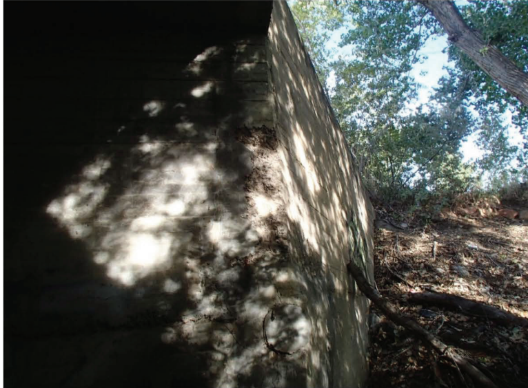
Spalling on southeast wingwall
