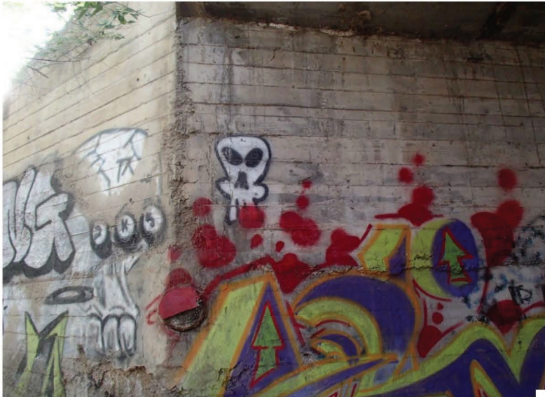
Crack with water leaking at southwest corner
