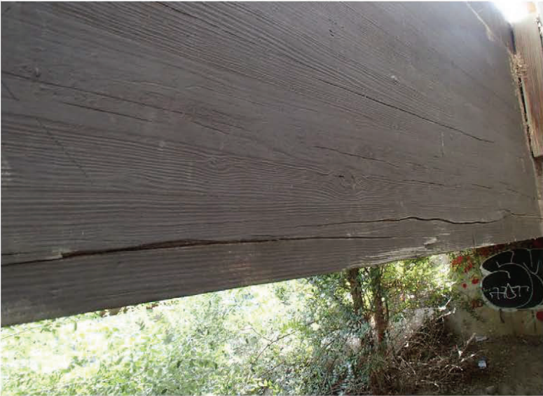
Check greater than 1 inch on girders
