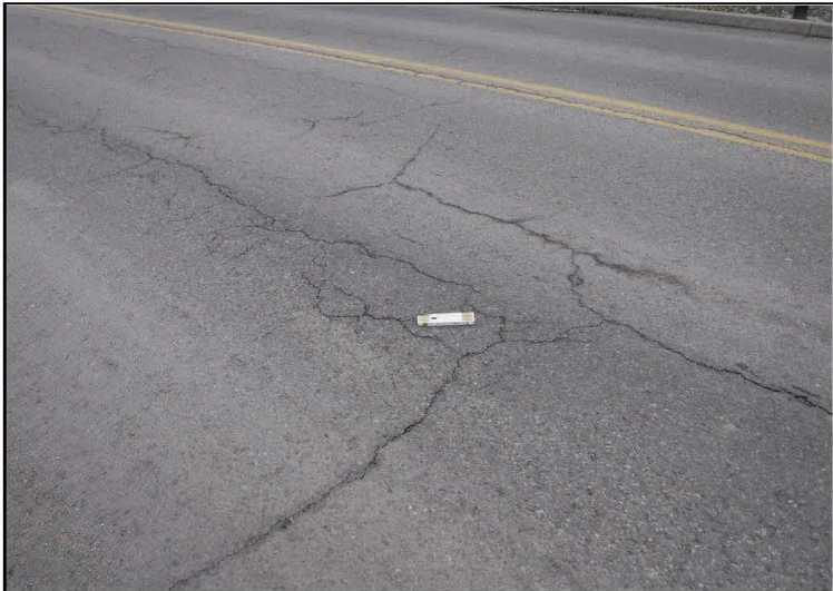
Map cracking in asphalt on top slab
