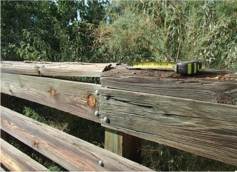
Weathered and rotting top rail
