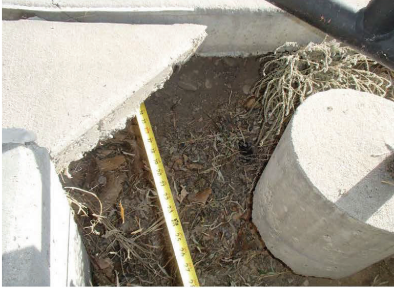
1.5 inch x 1 foot void under southwest sidewalk
