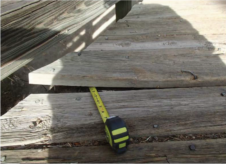
Protruding plank at northside
